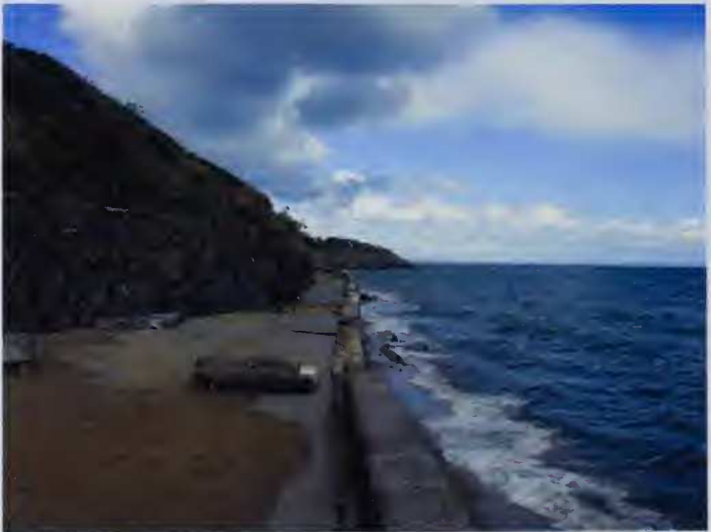
Fig. 5. Damaged sea wall south of Black Rock, 27 April 2009.
